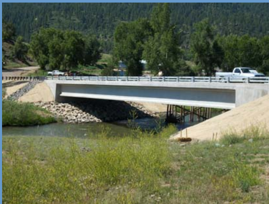
Juanita Bridge was one of the projects completed in the summer of 2009.
